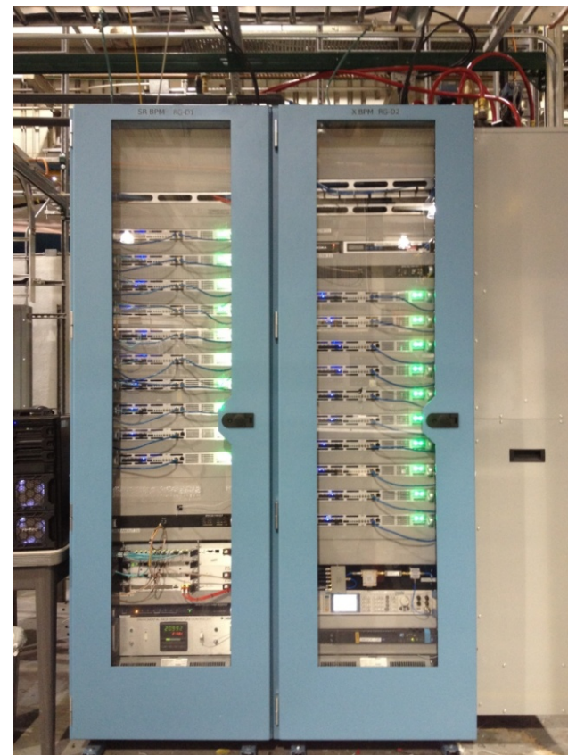
Storage Ring Thermal Racks Regulated to \pm 0.1\text{C}
